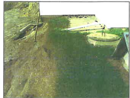
Washed away SSTS in eroded stream bank
