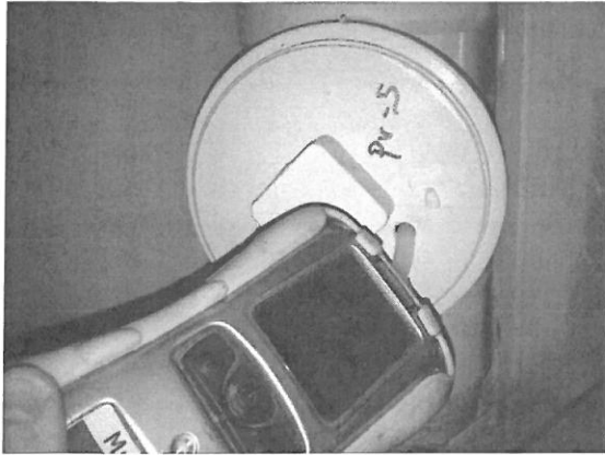
View of measuring for methane and LEL at the V-5 riser pipe for the passive venting system.
